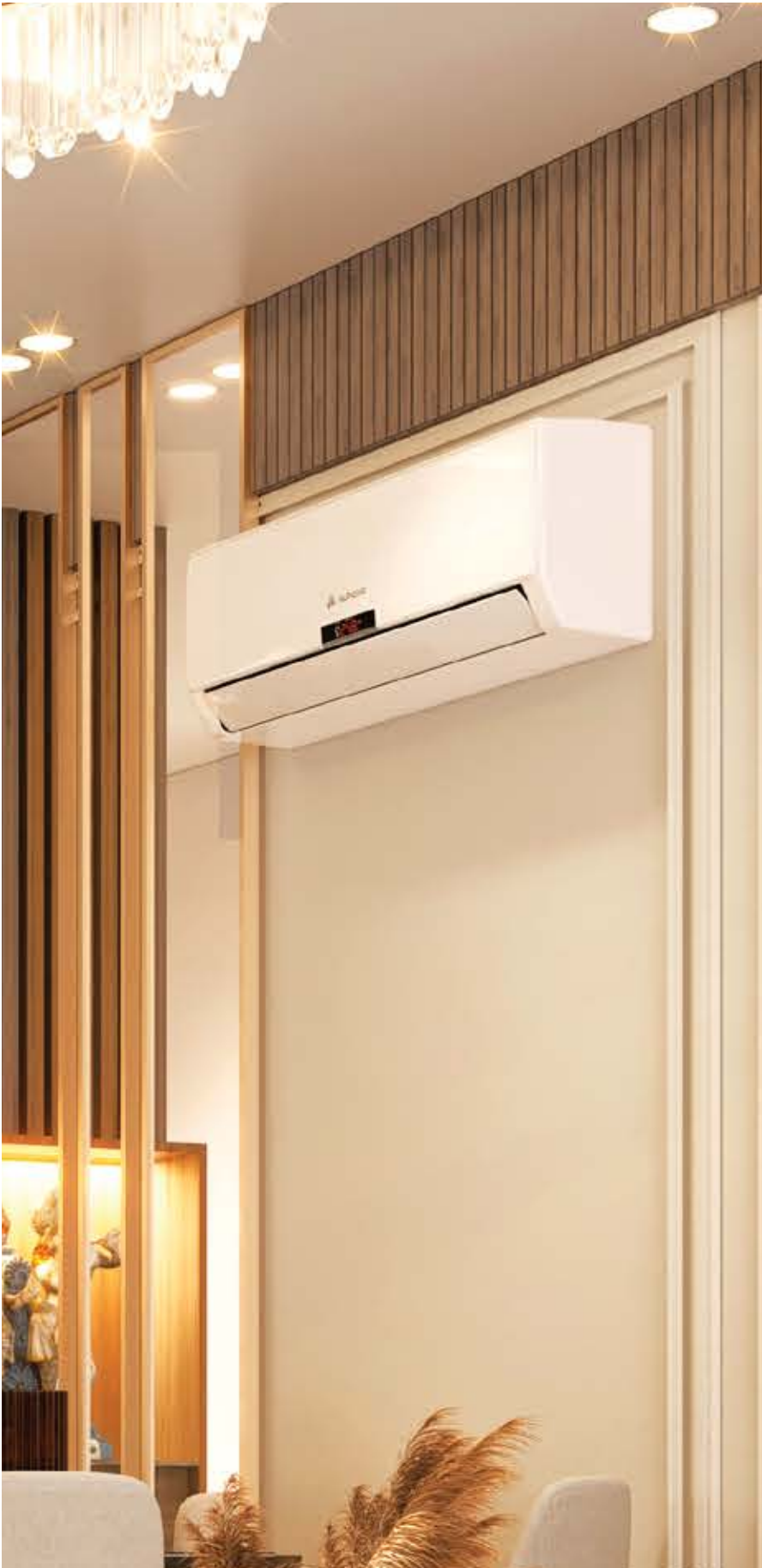
VRV/VRF Air Conditioning
